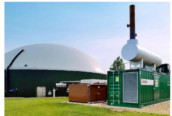
Courtesy of Clarke Energy
