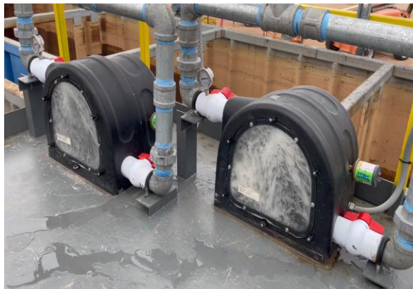
Energy storage demonstration / Generate electricity (March 2023)
